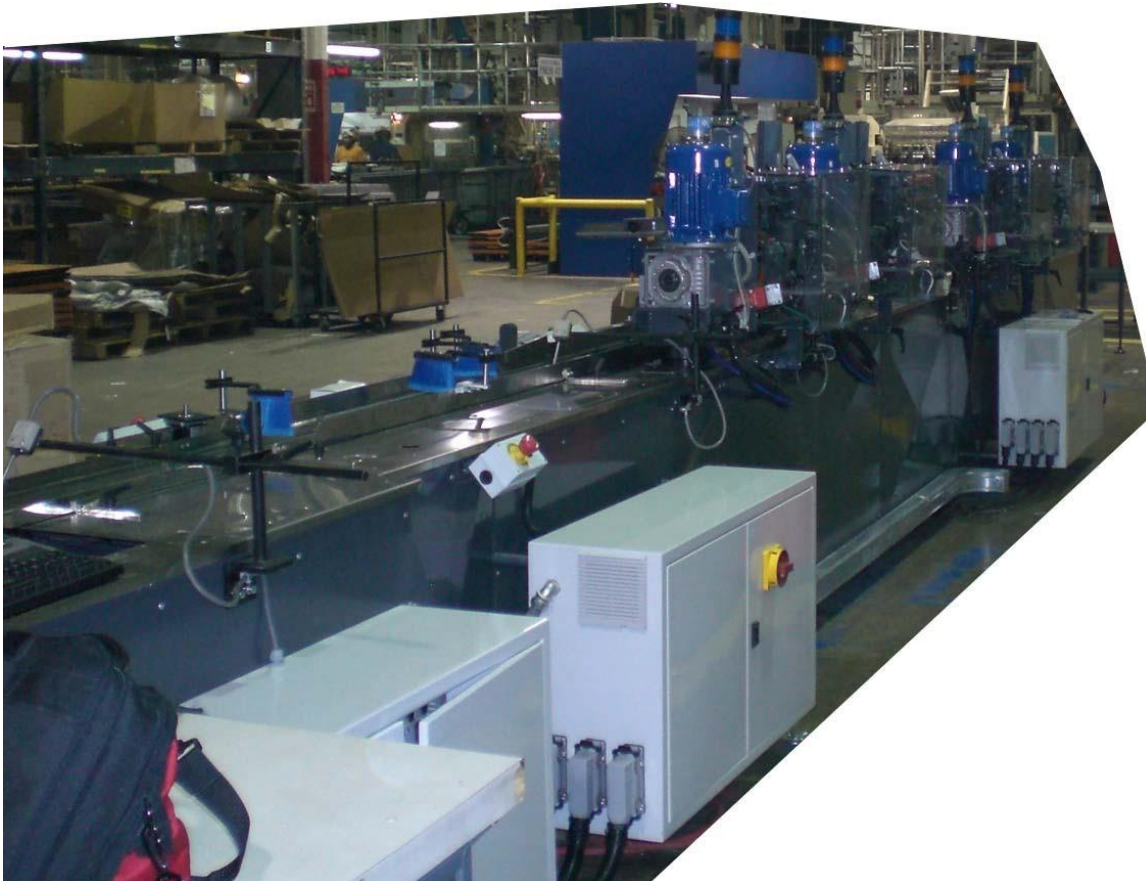
New electrical cabinets on SITMA gathering section
